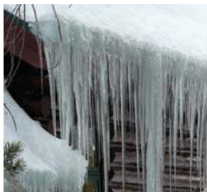
Unprotected roof and gutters
